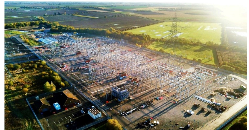
Electrical Substation at Bicker Fen, near Boston: similar scale to Navenby proposal
