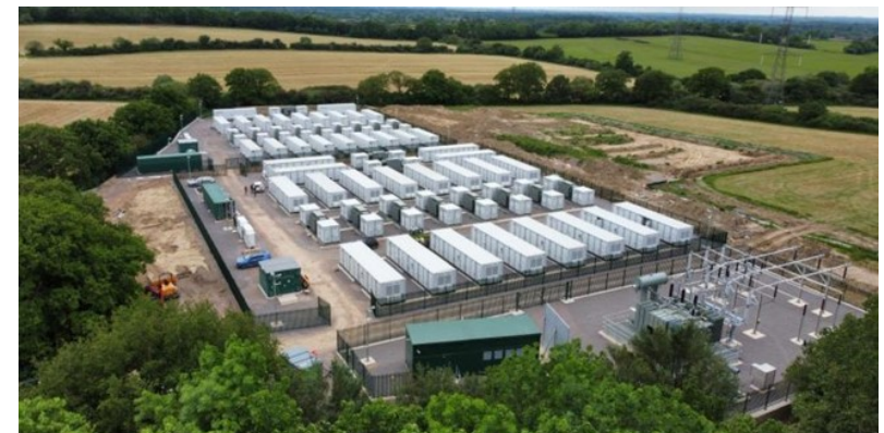
Battery Electrical Storage System at Kingston Upon Hull
